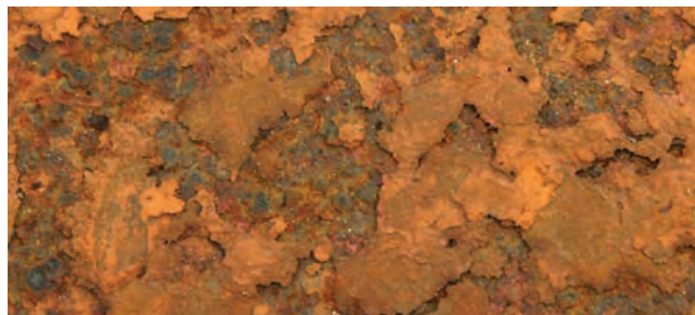
A close-up view of rust
